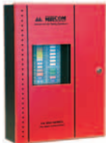
Conventional Fire Alarm
